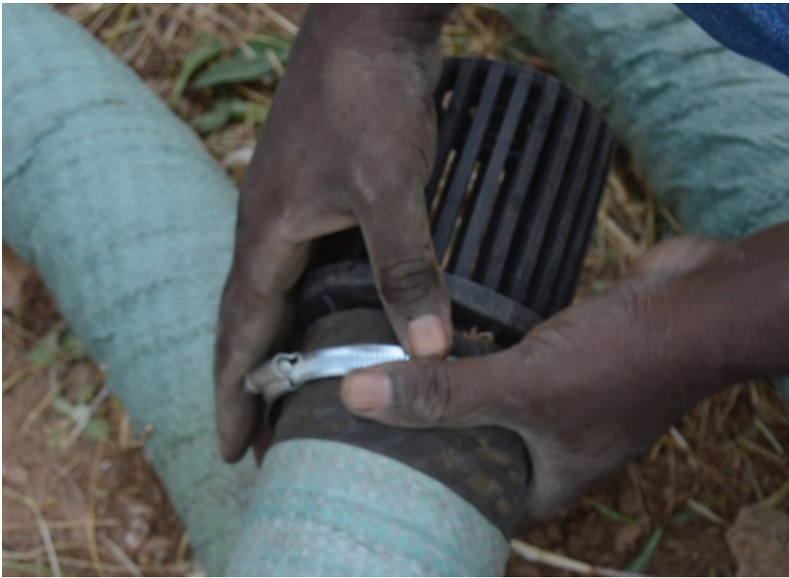
Fig 88. Inserting a strainer at the end of the suction pipe and tightening it with a clamp.
